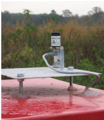
Figure 8: Photovoltaic sensor for measuring global radiation
