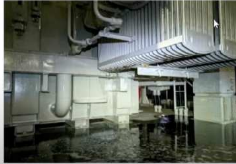
Transformer in Unit 1 leaked oil (Photo: Hokuriku Electric Power Co., Inc.)
